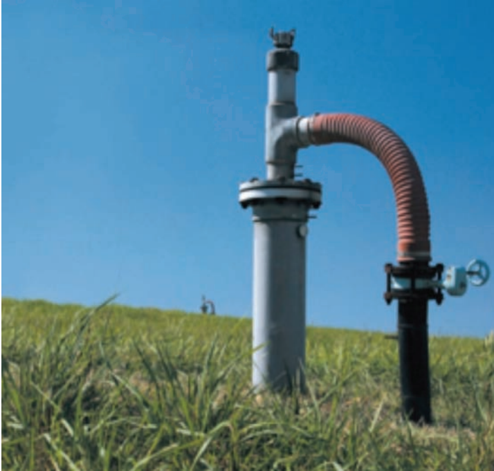
Pictured here is a well that is used to collect LFG on a landfill.
