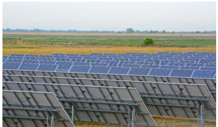
Davis Waste Water Treatment Facility solar array.
