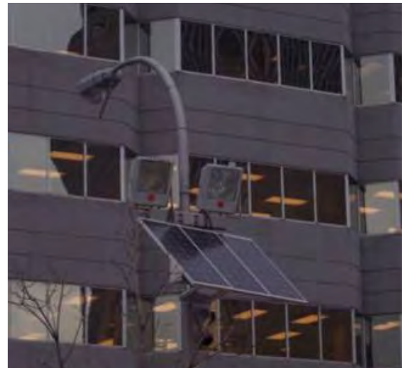
Figure 2. Another type of solar-powered streetlight.
