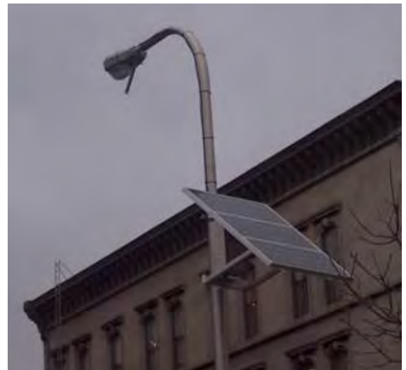
Figure 1. A solar-powered streetlight.
